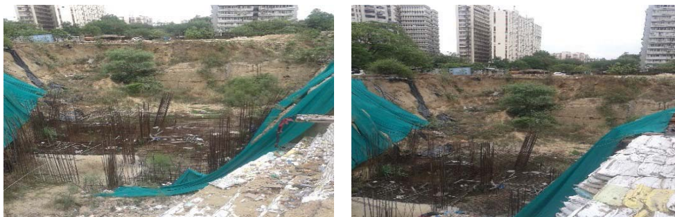
Construction work of MLCP at KG Marg stalled for want of ASI clearance
